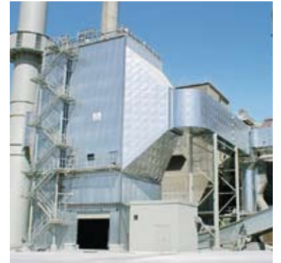
CEMENT WORKS, Germany PREHEATER KILN – MILL
