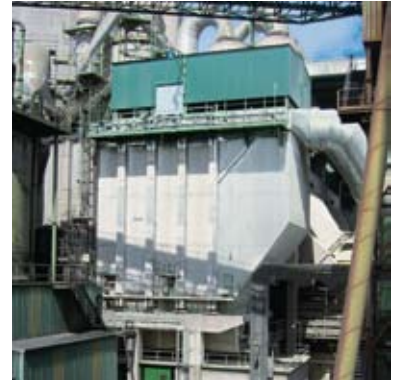
CEMENT WORKS, Spain PREHEATER KILN
