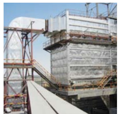
POWER STATION, India
