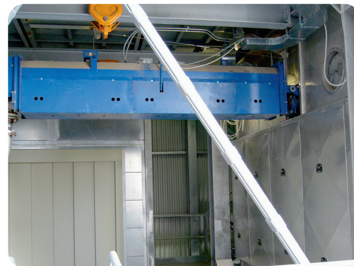
Catalyst layers with dust blower
