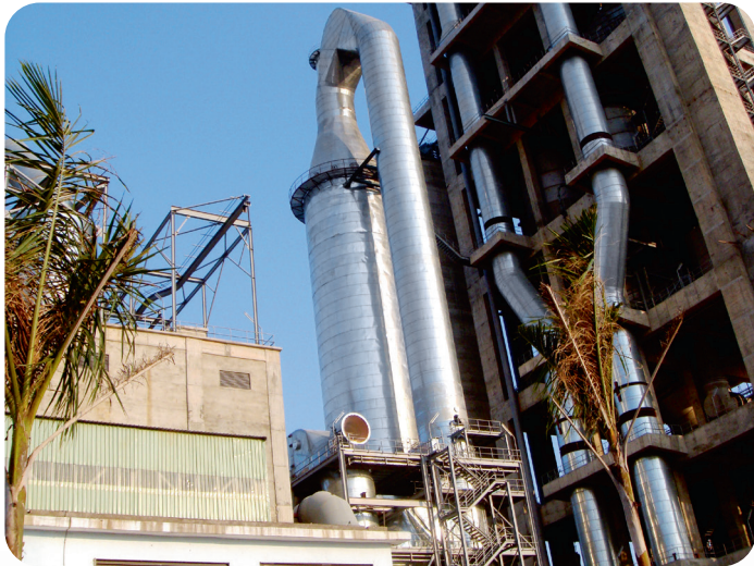
Cement works, Vietnam Preheater kiln
