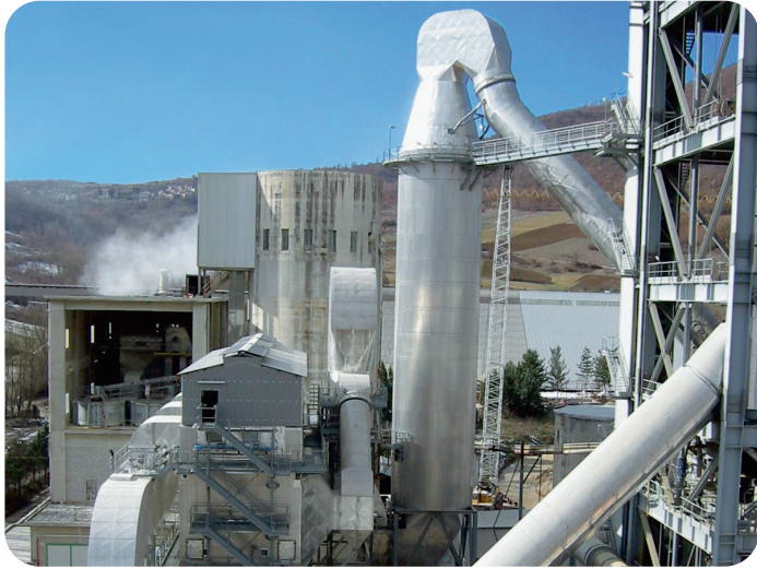
Cement works, Italy Preheater kiln
